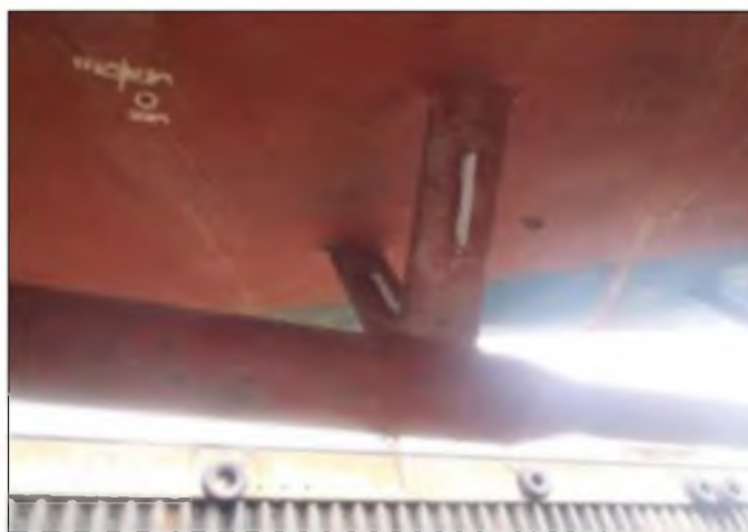
Figure 14 – Zinc anodes on the shaft brackets
